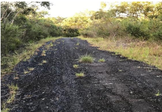
Deterioration in lower tarmac Rd
