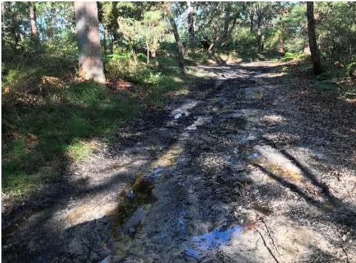
Some areas wash out after rain
